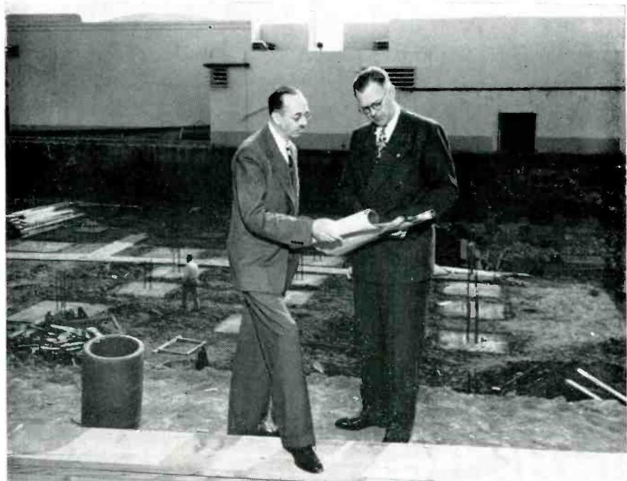
Mr. O. B. Hansen, NBC Vice-President and Chief Engineer, confers with A. H. Saxton, NBC Western Division Engineer, on the site of the new NBC additional studios at Hollywood Radio City, while in Hollywood on a week's trip to inspect the project.
